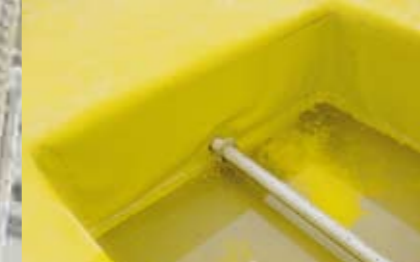
Garage roof deck with integrated tree planting box-outs; watertightness testing by flooding the plant boxes
