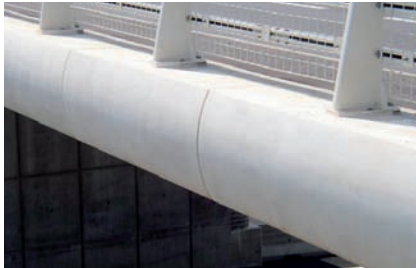
Fig. 8.9.4: Highly stressed building components such as columns and beams are made of high strength concrete. High resistance to external influences also makes high strength concrete an ideal protective coating for exposed construction elements.
