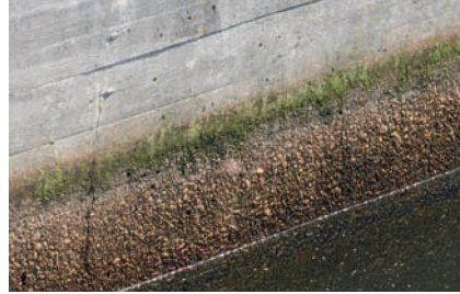
Fig. 8.8.1: Heavy leaching and damage to the structural concrete are observed particularly in the water splash zone of biological treatment basins.
