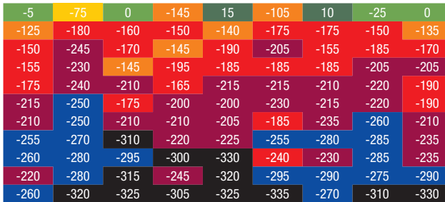
Fig. 8.2.4: Potential measurement on a retaining wall along a road with heavy traffic with high use of de-icing salt, after less than 10 years of exposure. The darker the coloration, the higher the potential for corrosion.
