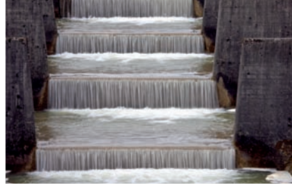
Fig. 8.7.1: Particularly in whitewater, concrete surfaces are subject to massive additional strains by rubble, sharp edges and abrasion, as well as possible temperature stresses due to frost exposure.
