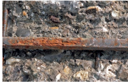
Fig. 8.2.1: Damage to concrete structure due to insufficient concrete cover and low concrete quality.
