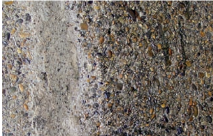
Fig. 8.7.5: Due to continuous exposure, the cement film is eroded in an initial step, and thereafter larger and larger aggregates are rubbed, knocked or washed out of the hardened cement paste.
